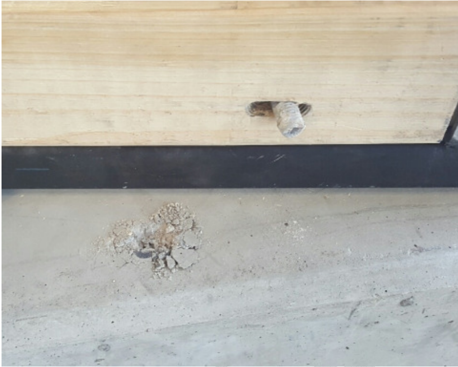
Figure 18: Anchor in shear failure (zoomed in)
